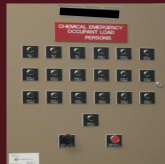
Enhanced Shelter In Place (ESIP / CPS) Control Panel
